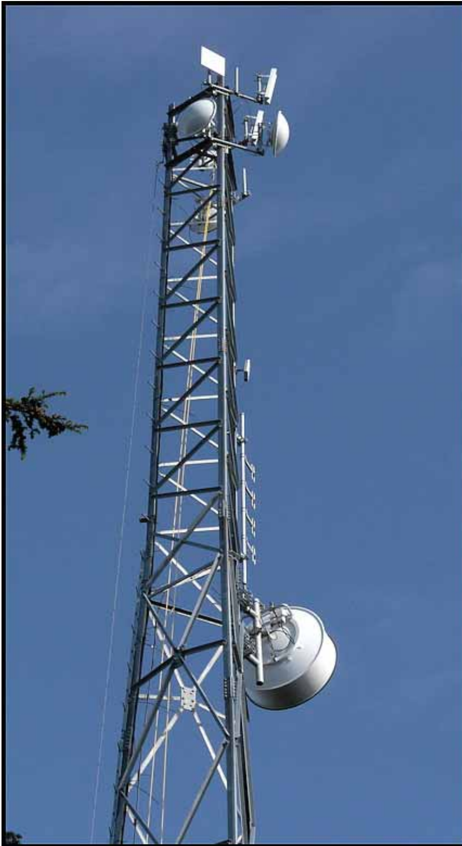
GBIS tower on Pocahontas - large Parksville link dish for ambulance service of BC below with ham radio antenna above it. The top section has internet radios only.
