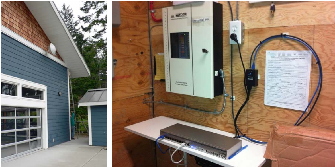
The dish at SCHC and the GBISoc equipment and the Telus cable.
