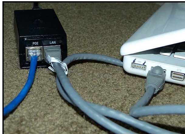
Bypass Router. The black injector box is connected directly to a laptop, computer, etc. , grey cable from LAN socket. The blue cable goes from the injector box [POE socket] to the white box or dish (the Internet radio) outside the house. Turn your router off for this test.
