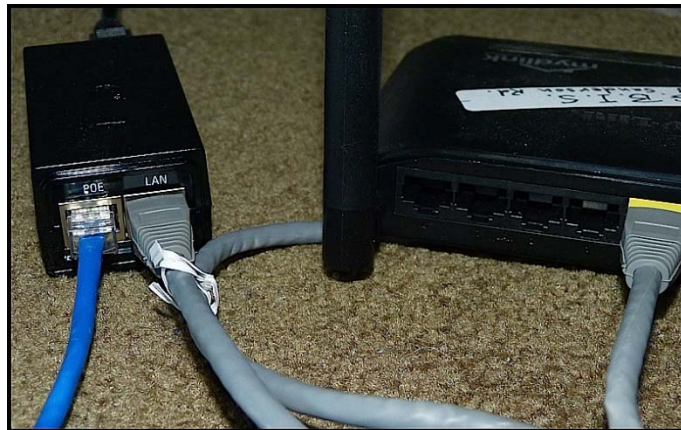
Router on. The black injector box is connected to the back of a home WiFi router , grey cable from LAN socket. The blue cable goes from the injector box [POE socket] to the white box or dish (the Internet radio) outside the house.
