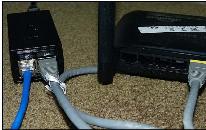
Router on. The black injector box is connected to the back of a home WiFi router , grey cable from LAN socket. The blue cable goes from the injector box [POE socket] to the white box or dish (the Internet radio) outside the house.
